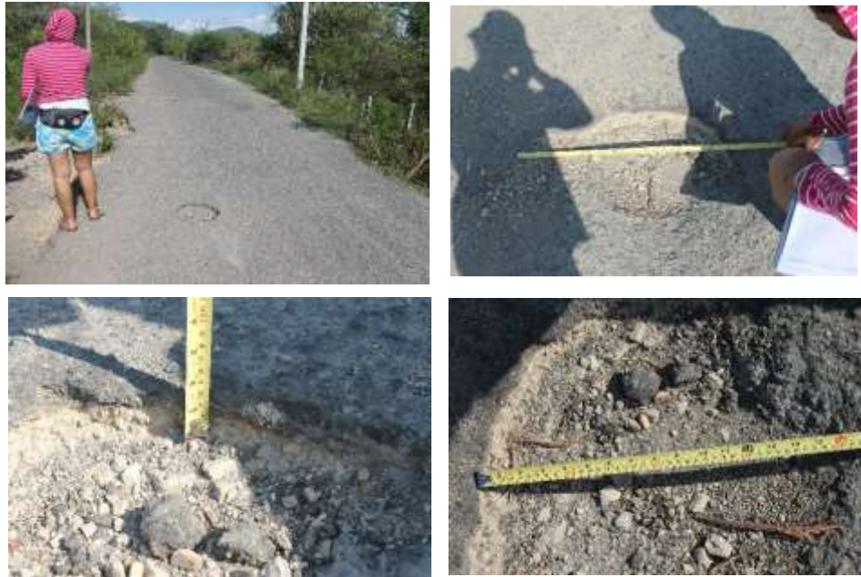
Figura 4. Falla 2 Bache (Km4+958,35)
