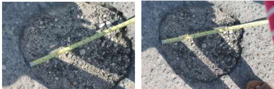
Figura 5. Falla 3 Bache (Km4+954,34)
