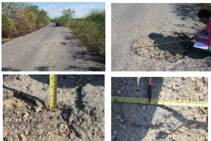
Falla 8: Bache (Km2+860)
