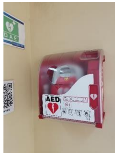
Prevention Equipment, (Building...)
