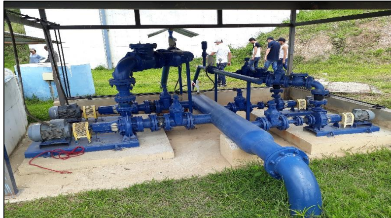
Figura 20. Fotografía bombas RAS - WAS
