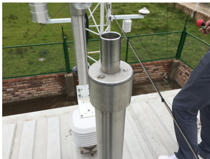
Fig#6: Arreglo fuga PM2.5 Nazareth.
