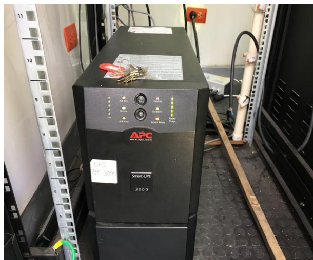
Fig#10: UPS Paipa.
