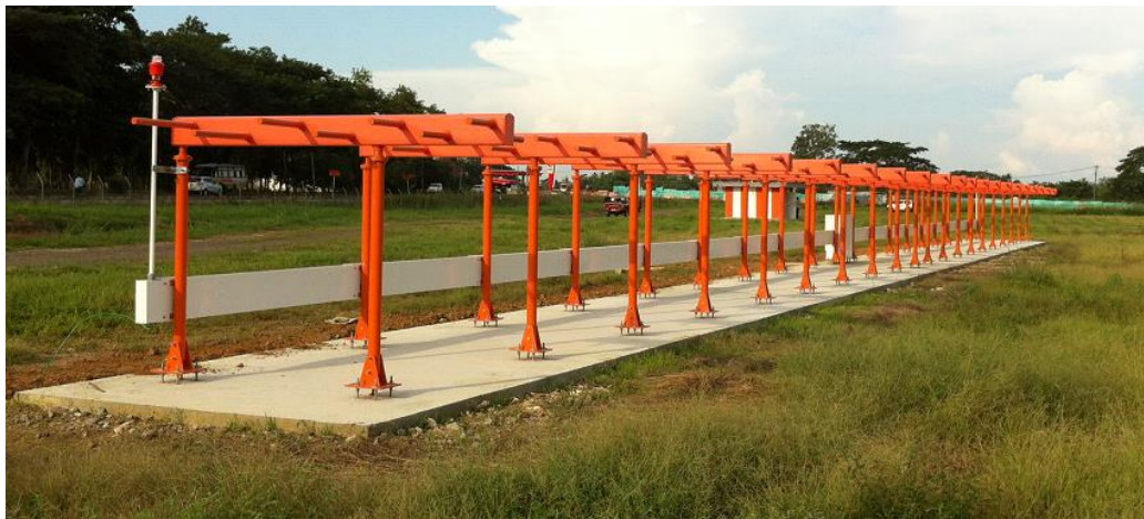
Figure 1-14. Typical 20/10-LPDA installation
